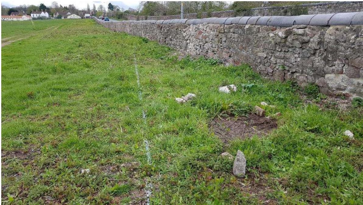
CR6 – approximate line of rebuilt stone wall set-back to allow for over-run area for large vehicles exiting left (new compound vehicle entrance behind viewer).
