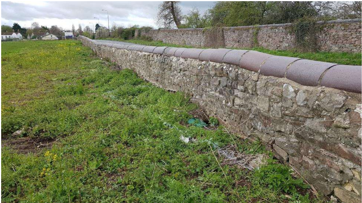
CR4 – proposed new separate permanent landowner access with walls rebuilt and setback for visibility.
